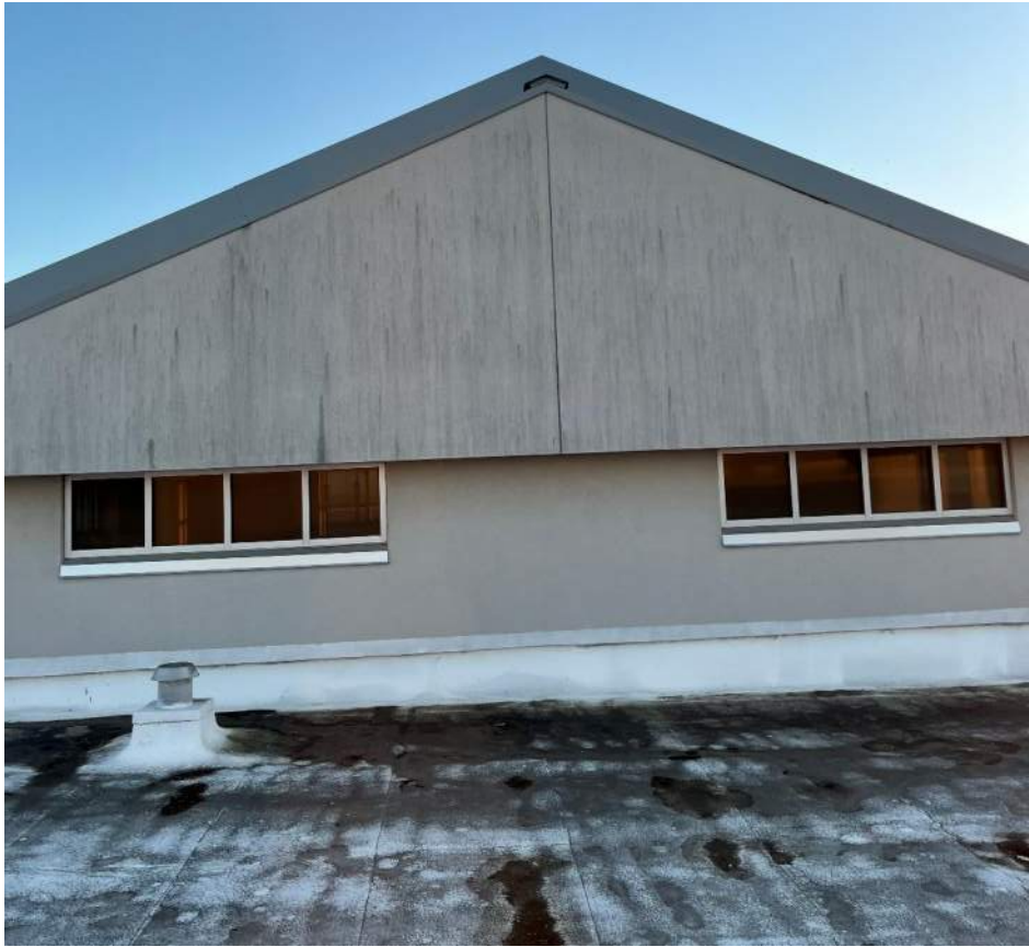
Staining of EFIS Walls
