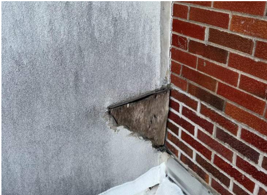
Damaged EFIS Wall
