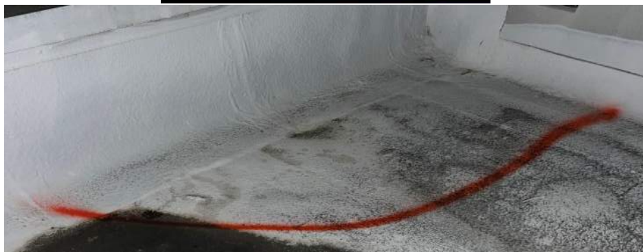
Larger Wet Area in SPF Foam Roof Assembly.
